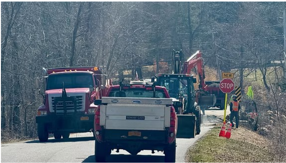
Work crew covering newly installed pipes beneath Oscaleta Road on Wednesday. THANE GRAUEL PHOTO
