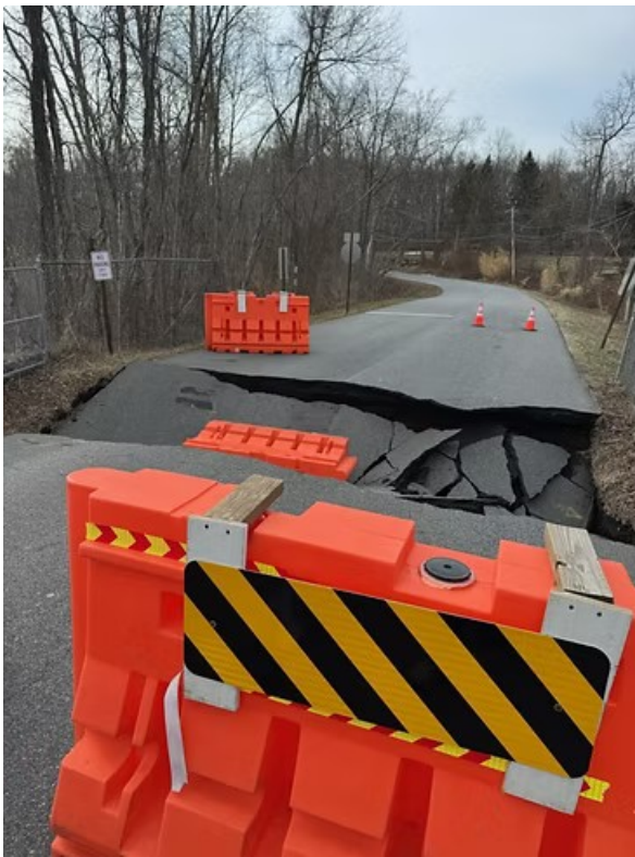
Oscleta Road after the culvert collapse on Sunday. TOWN OF LEWISBORO PHOTO
