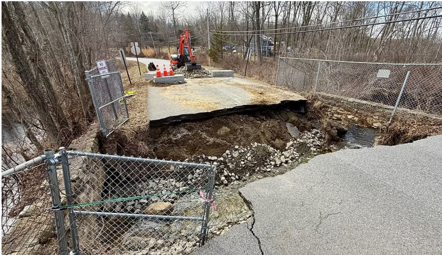
The culvert under Oscaleta Road after debris was cleared and a channel carved. THANE GRAUEL PHOTO
