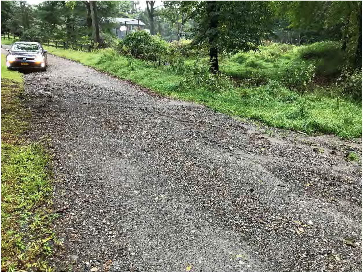
Figure 71 Gully erosion and runoff of materials on Old Pond Road (Sites 7 & 8)
