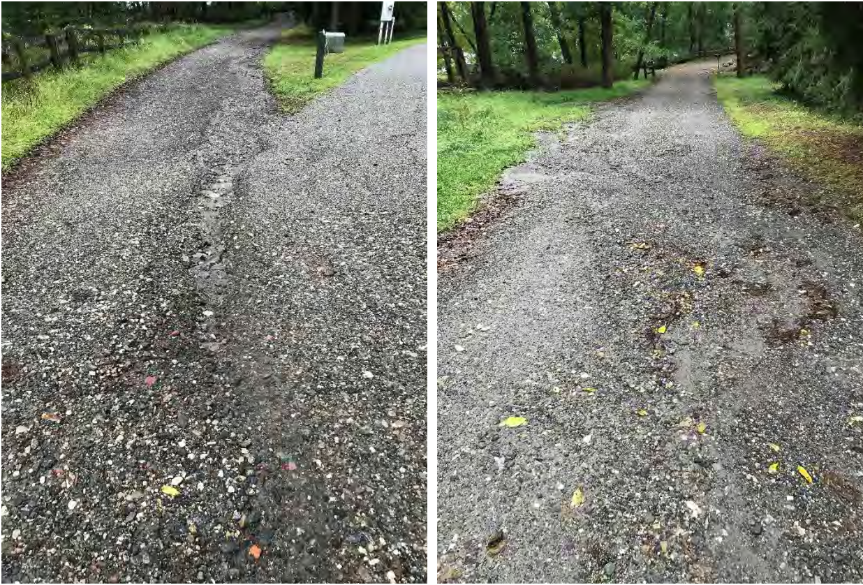
Figure 70 Gully erosion on Old Pond Road (Sites 7 & 8)
