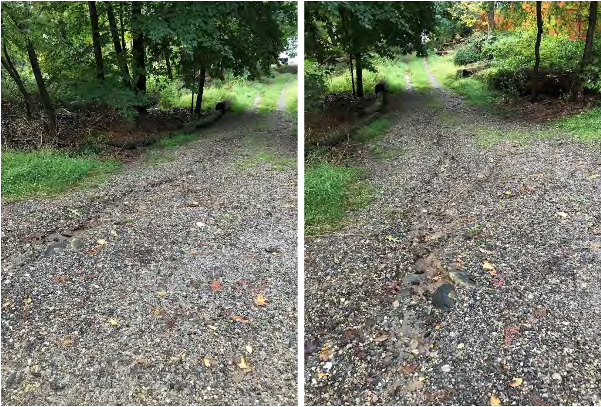
Figure 74 Gully erosion on private launch off Old Pond Road (Site 11)
