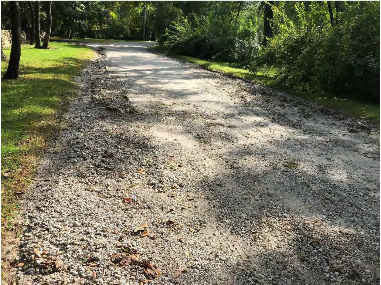
Figure 78 Photo of road scour and erosion on East Ridge Road (Site 24)
