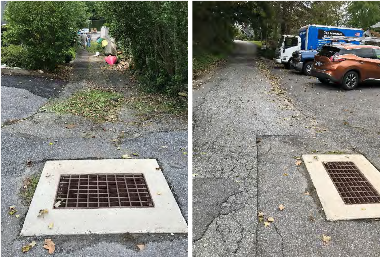
Figure 84 Collapsed storm drain and overland flow into Lake Waccabuc on Cove Road (Site 2)
