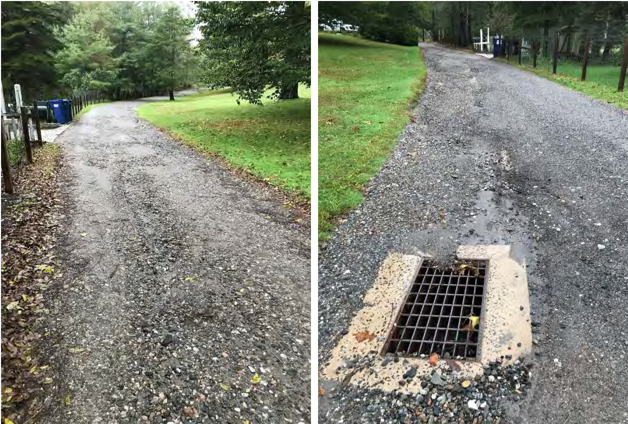
Figure 68 Gulley erosion and runoff entering storm drain on Old Pond Road (Sites 5 & 6)
