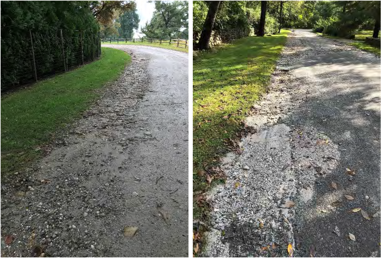
Figure 77 Photo of road scour and erosion on East Ridge Road (Sites 21 & 24)
