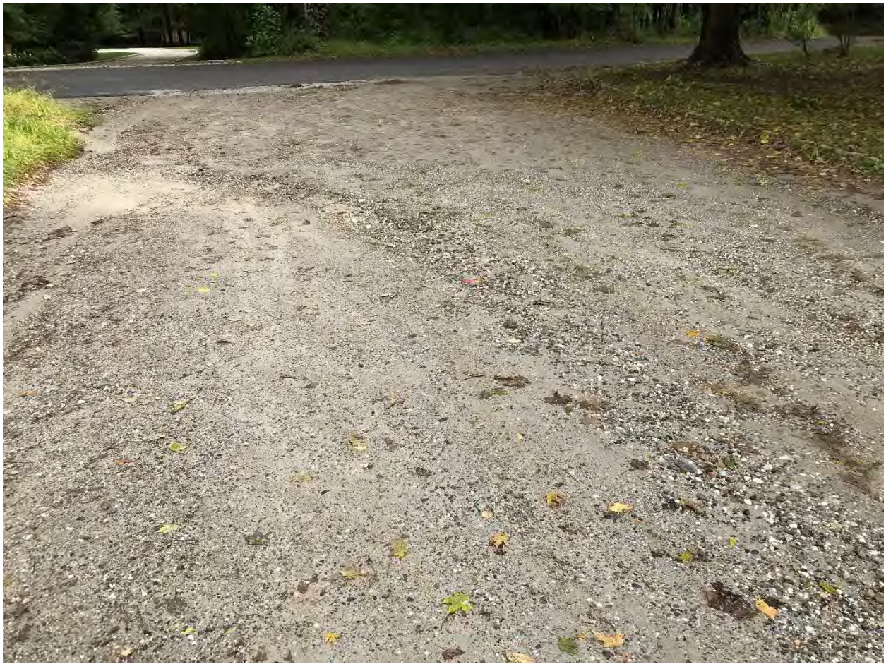
Figure 75 Photo of road scour and erosion on East Ridge Road (Site 20)
