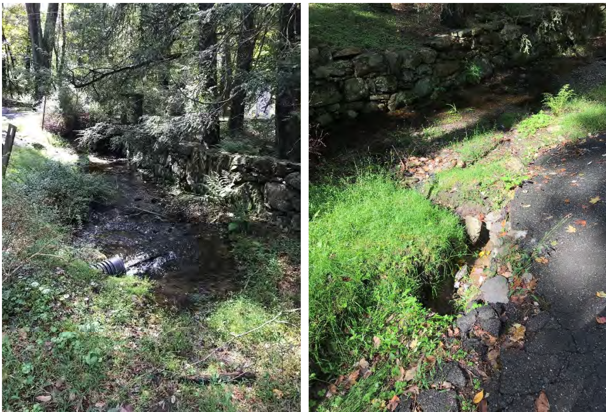
Figure 87 Photo of roadside erosion into stream on Oreneca Road (Site 31)
