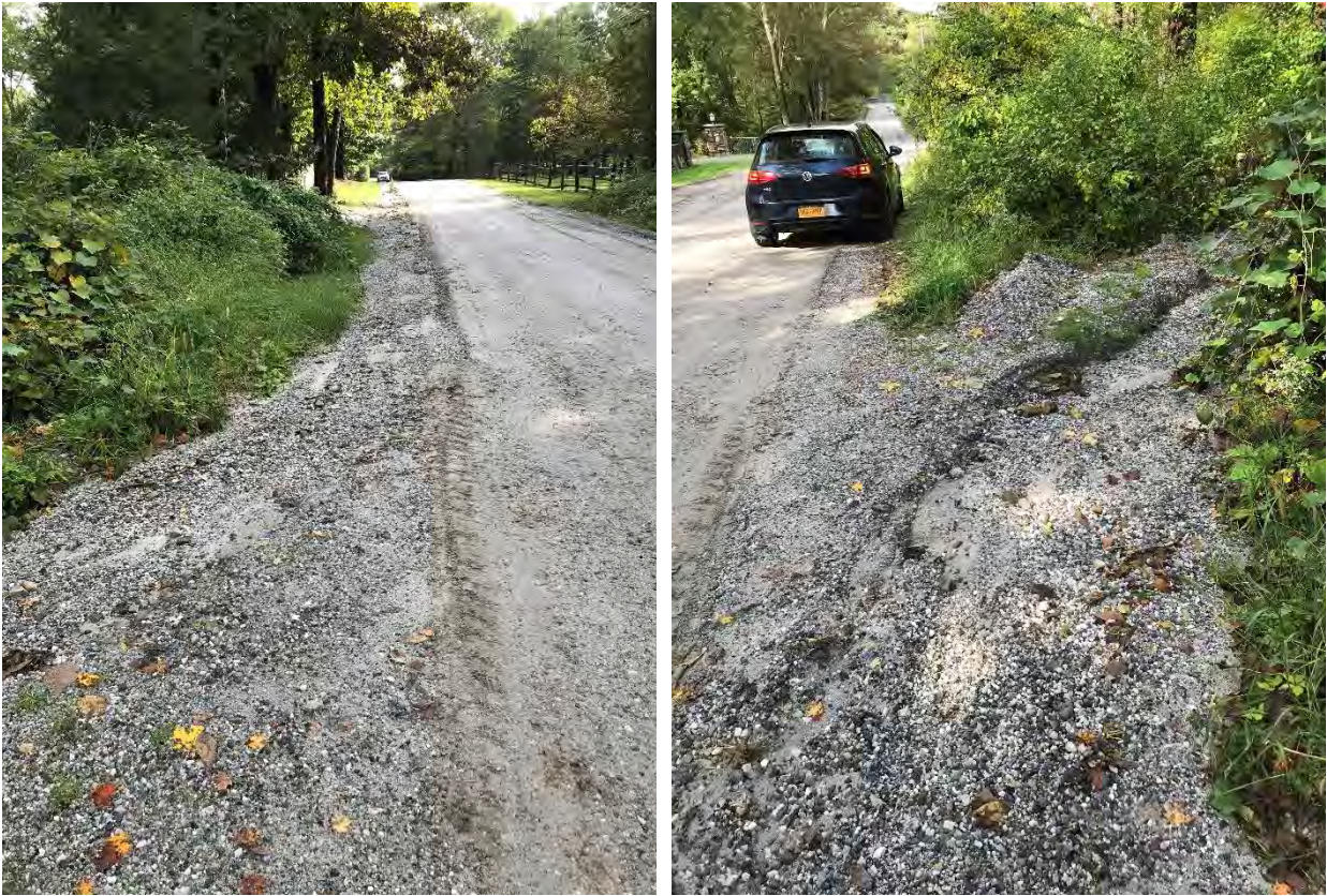
Figure 79 Photo of road scour and erosion on East Ridge Road (Sites 25 & 26)
