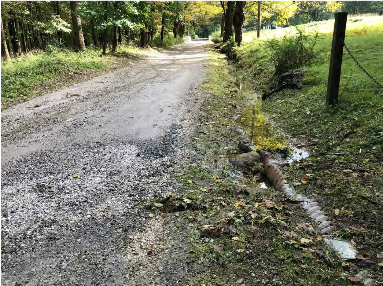
Figure 66 Photo of erosion on Tarry-A-Bit Road (Site 4)
