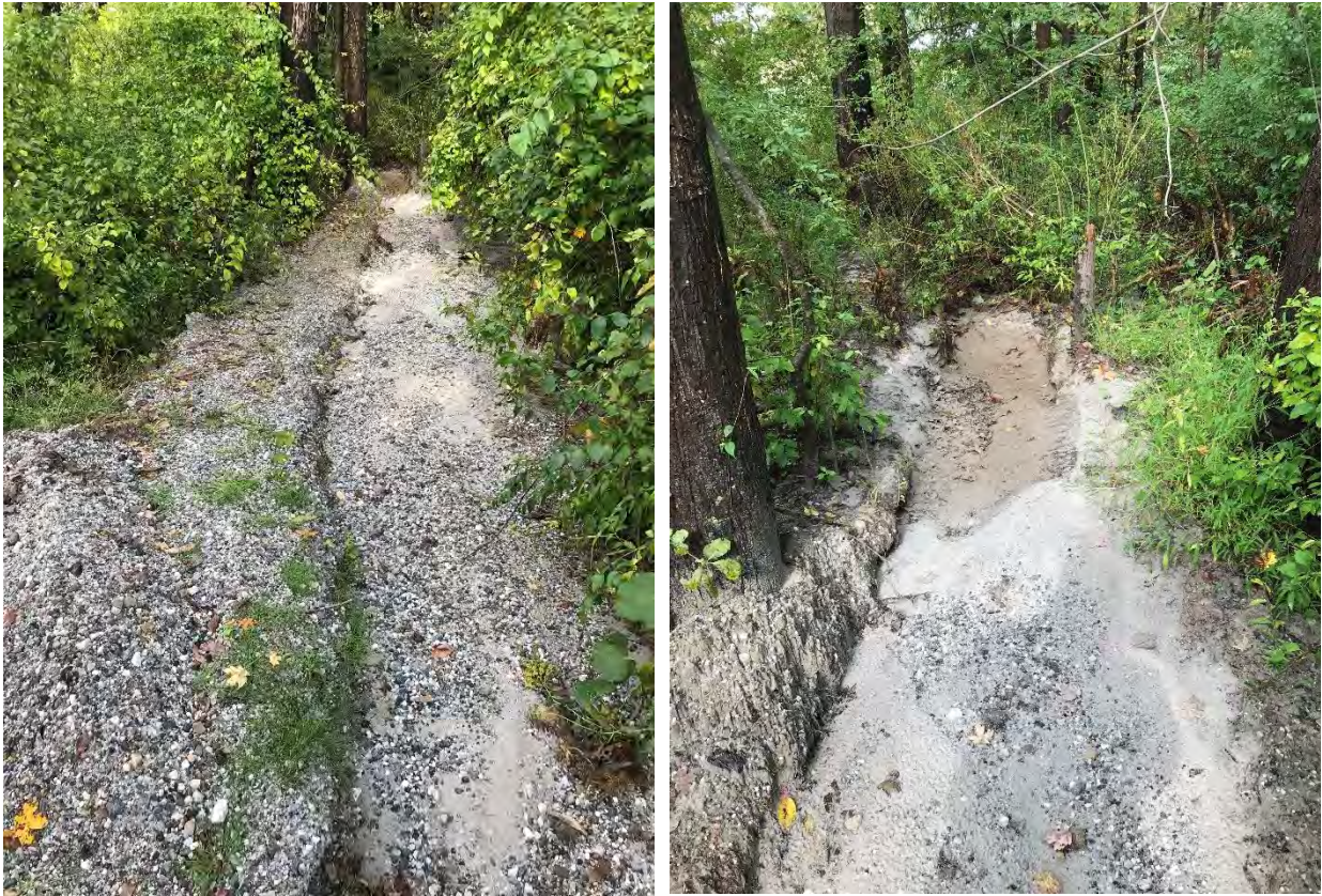
Figure 80 Photo of material runoff from erosion on East Ridge Road (Sites 26 & 27)
