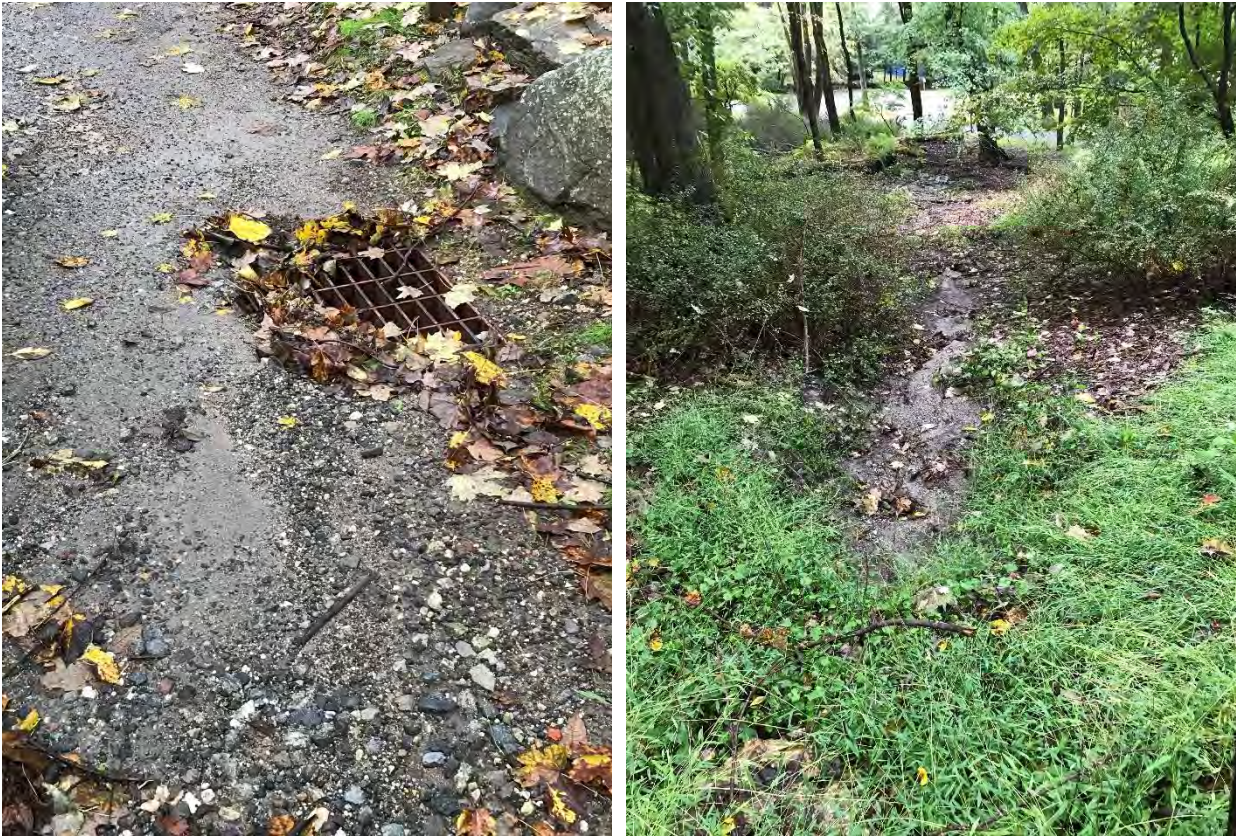
Figure 72 Clogged storm drain and runoff of road material on Old Pond Road (Sites 9 & 10)
