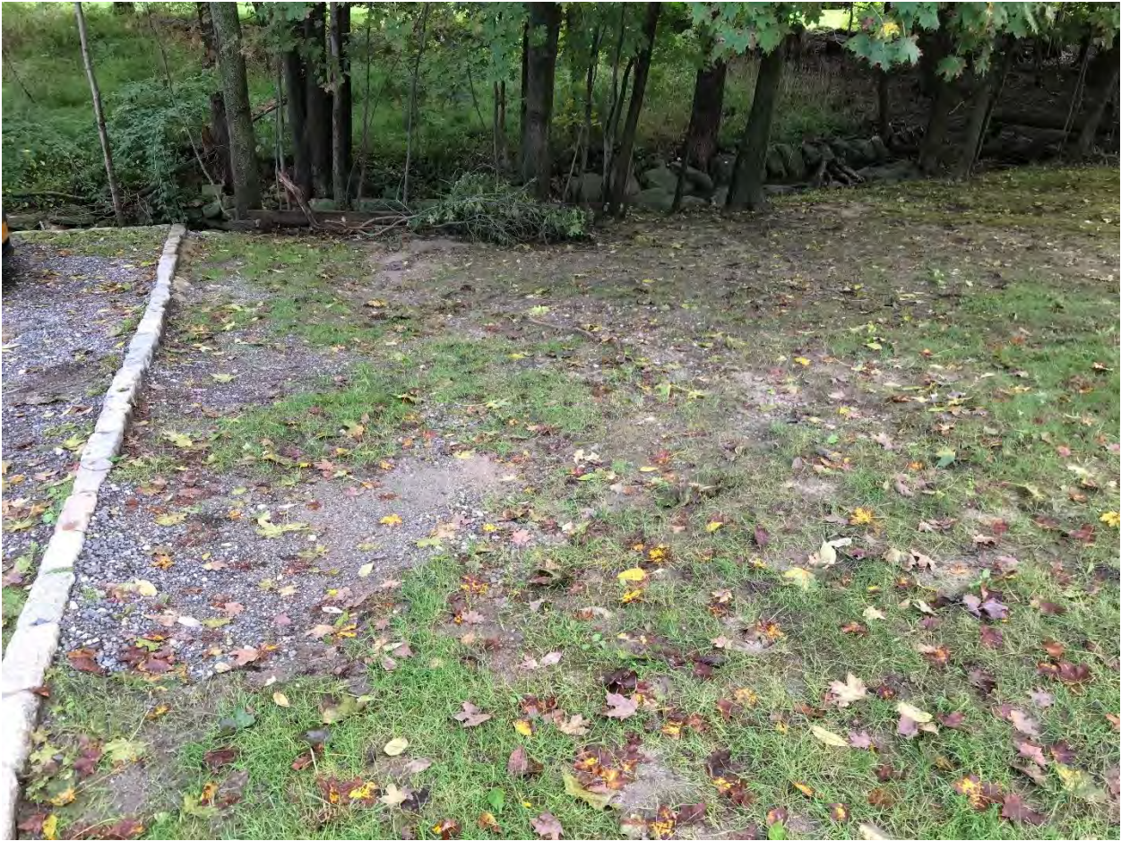
Figure 85 Runoff and erosion from Post Office parking lot and Mead Street (Site 29)
