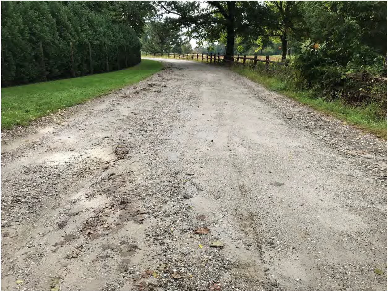
Figure 76 Photo of road scour and erosion on East Ridge Road (Site 20)
