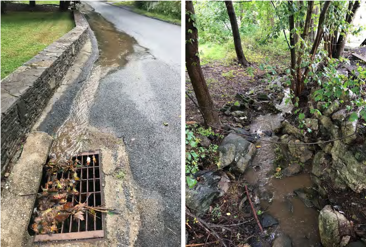
Figure 83 Runoff from roof/lawn carrying silt along road into storm drain and stream channel (Site 12)
