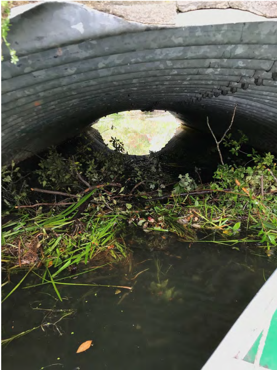
Figure 65 Photo of plugged culvert due to beaver activity (Oscaleta-Waccabuc channel)
