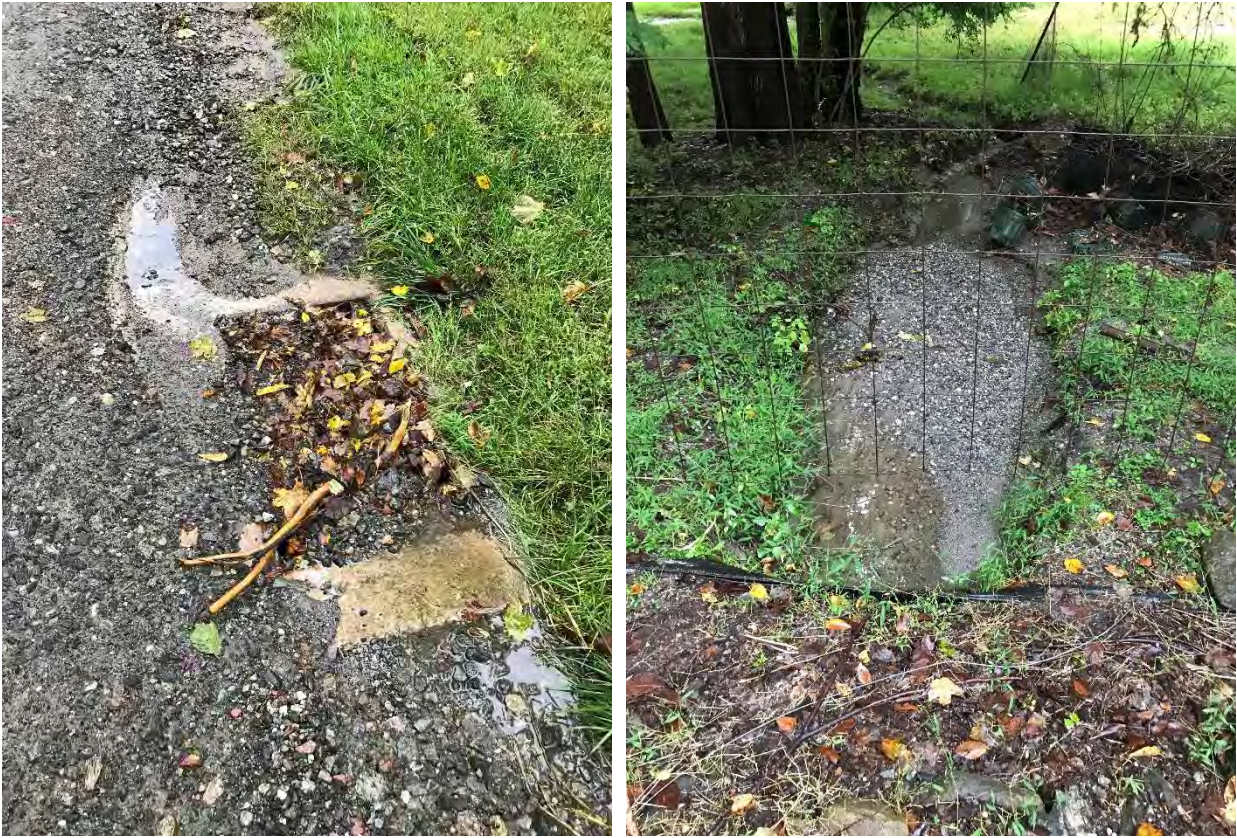
Figure 69 Clogged storm drain and road material washing into drainage ditch on Old Pond Road (Sites 5 & 6)
